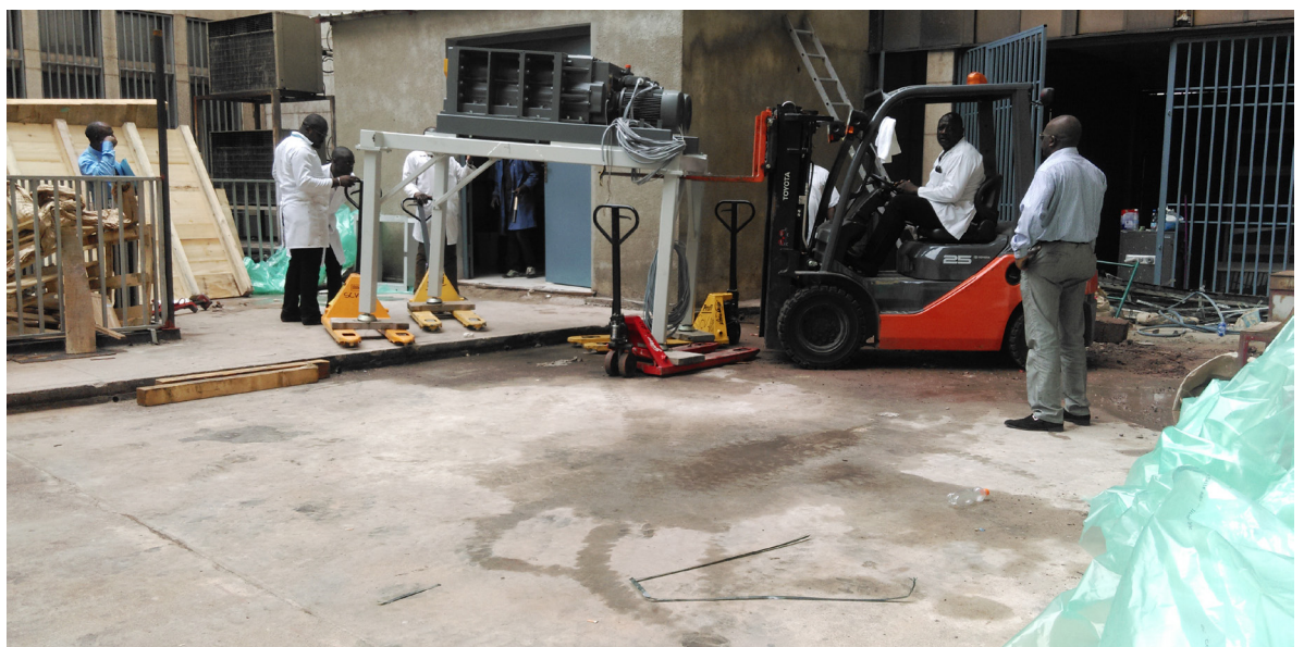
After the success of the first bank note destruction system for Kinshasa, the Central Bank of the Congo ordered a second for Kisangani in the north-east of the country.
